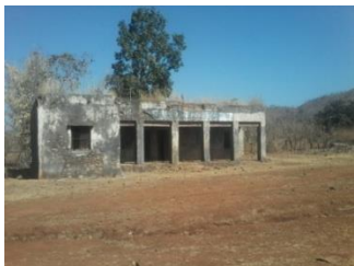
Dilapidated School Building, Bhuri Talai
